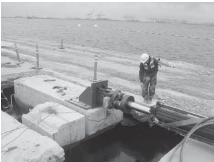
The metal pole is an “actuator,” a giant hydraulic piston. With great force, it pushes against the side of the pier. Photos: UC San Diego, Department of Structural Engineering
